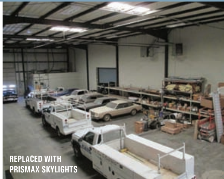
OLD TRANSLUCENT SKYLIGHT PANELS
