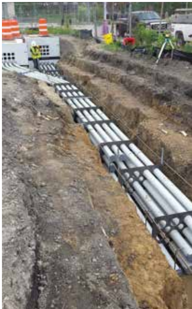
Motor City Electric worked on the Quicken Loans Technology Center, a 66,000-square-foot data center and office complex in Detroit. MCE's fab shop produced the conduit spacers for the duct bank, which helped cut costs and increase productivity.
