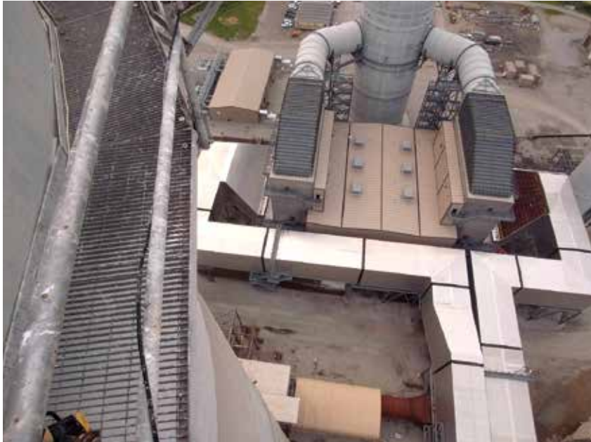
Sachis is performing the balance of the upgrade at Newton Power Station, including all electrical installations.
