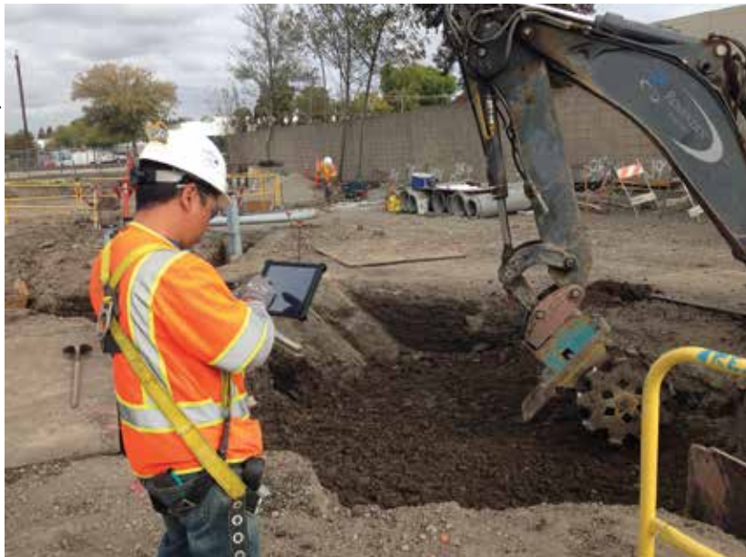
This Rosetini Electric electrician is using mobile technology on the 10-mile BART extension project into Santa Clara Valley. The new line will connect the existing Fremont Station to a new station in Milpitas and terminate at the first San Jose BART Station, Berryessa.
