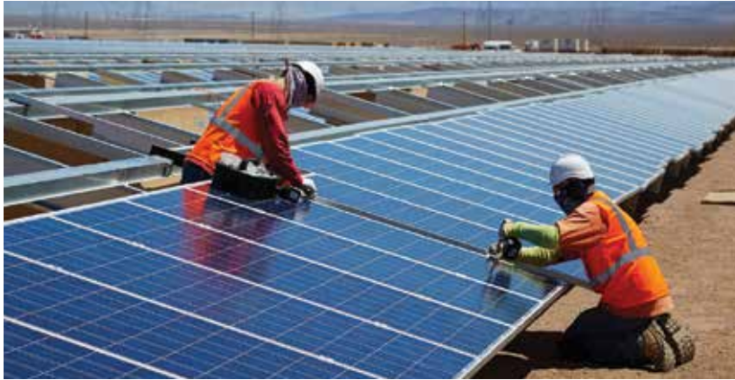
Cupertino Electric employees installed a large number of solar panels at the Copper Mountain Solar 3 project in Nevada.
