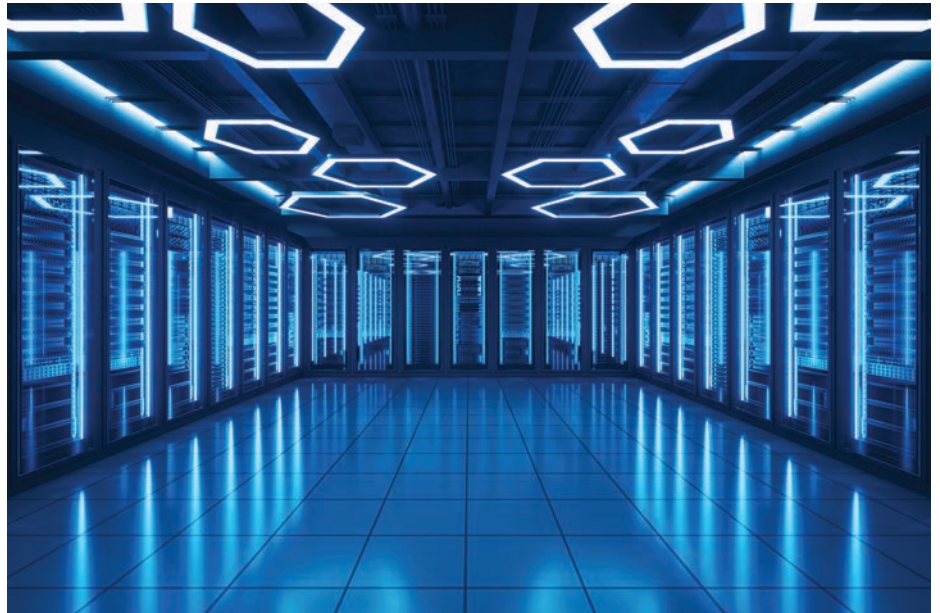
Technological advances are allowing data centers to be built in more diverse locations across North America.
