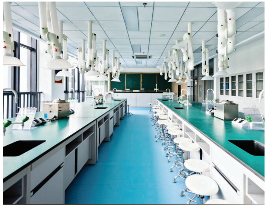
Specialized equipment and plumbing are part of many life sciences facilities.
