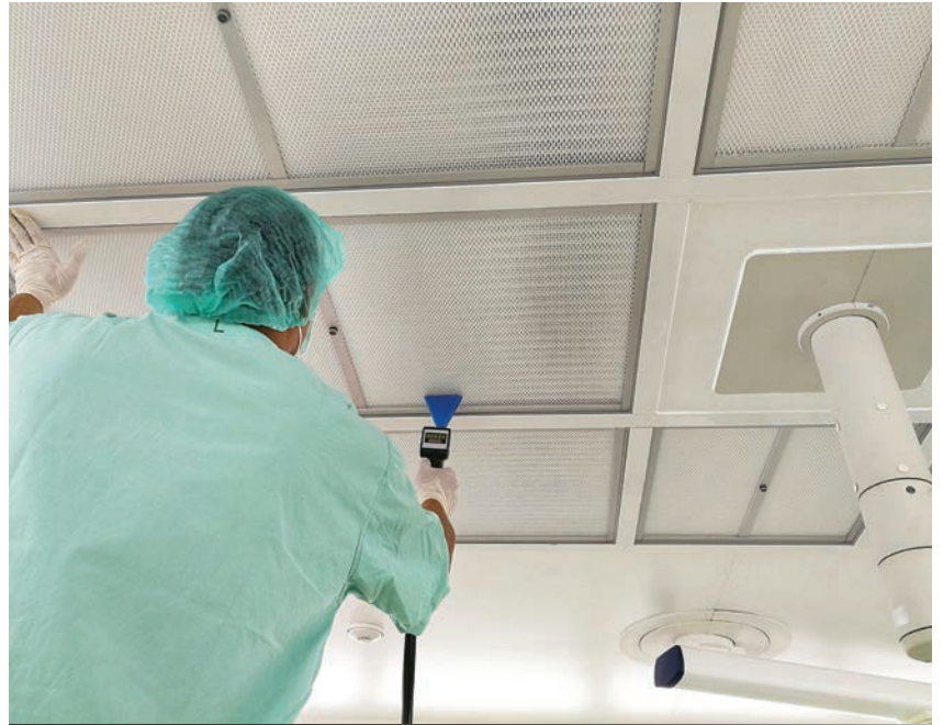
HVAC systems in a life sciences cleanroom must meet strict standards, including HEPA filtration.
