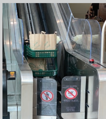
SAFETY GATES OPEN ONLY FOR CARTS
