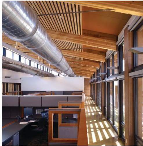
Inverted king-post trusses with laminated wood beams offer a high strength-to-weight ratio and exceptional ductility for improved structural performance during times of strong desert winds or seismic events.
