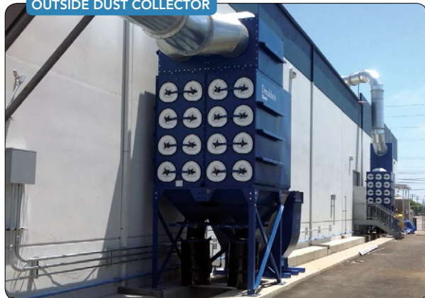
Figure 2. Locating the collector — in this case, equipped with explosion venting and isolation valves — on the exterior of the process area may make sense.
