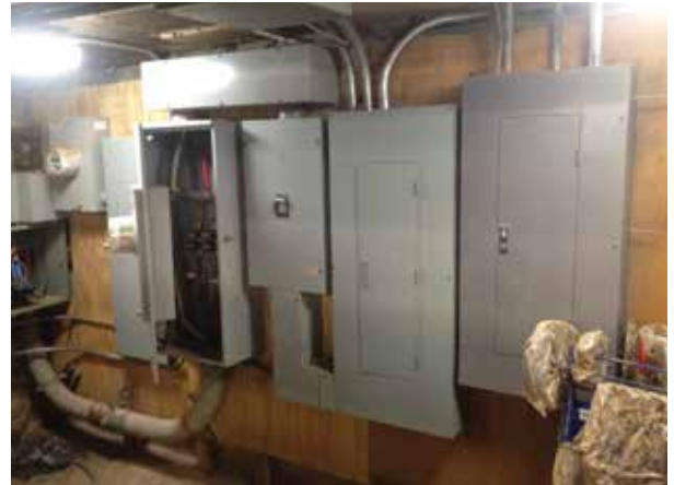
This equipment was completely submerged in salt water and left in service. Photo by Jack Lyons
