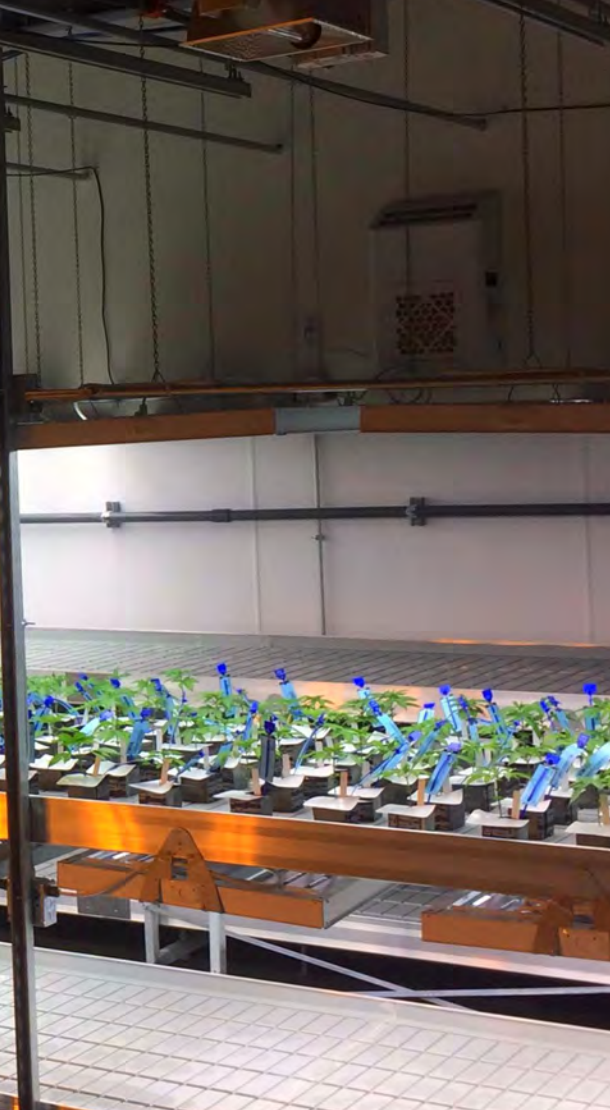
(Left) Two technicians inspect the young plants in the double-stacked T5 area of the veg room. (Right) The Priva touch points [similar to an iPad] outside each room give current readings for temperature, humidity, CO 2 , fan speeds, and more, and enable growers [with high enough security clearance] to review history and/or make needed adjustments.
